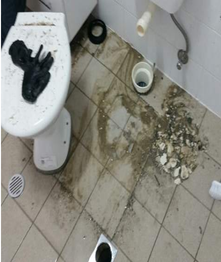
Cleared main line blocked due to rocks and sand in the line from construction
